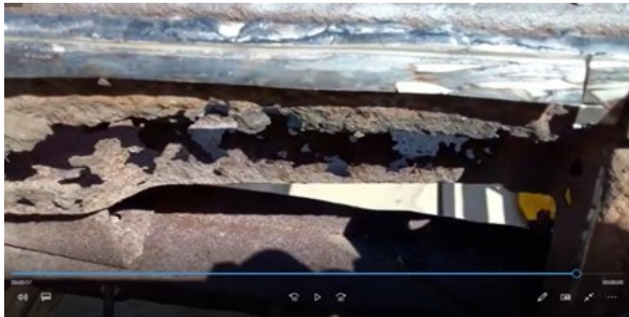
Above: The badly rusted frame to which some of the body parts were welded to.
