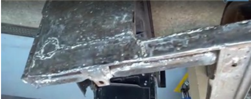
Above: The body is turned upside down to repair the badly welded panels and replace some of the frame sections.
